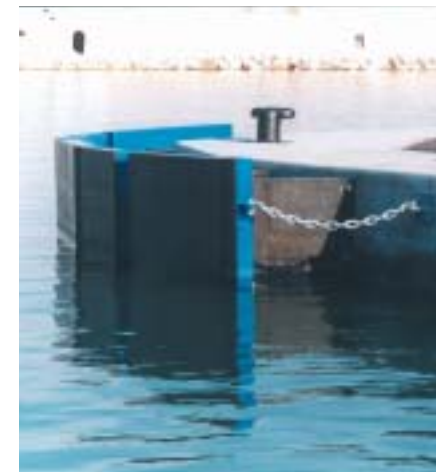
▲ Corner Fender, Marseille (FRANCE)
